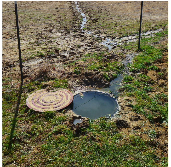
MDB engineer assessing soils in Gallup, NM (top), and Wastewater seepage at residential septic system in Gallup, NM (above).
